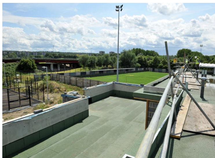
Sporting Club Thamesmead takes shape with the multi-use games area (left), main pitch (centre) and the new pavilion under
